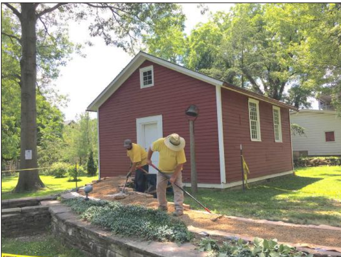
Thanks to a grant from The Nord Family Foundation, OHC was able to hire Locke's GoGreen to resurface the pea gravel path to the 1836 Little Red Schoolhouse.
