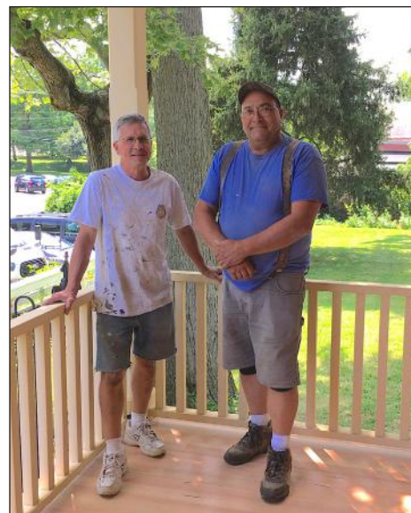
Scott Broadwell and Pat Ives teamed up to floor and paint the rear porch of the Monroe House and bring it back to its former glory.
