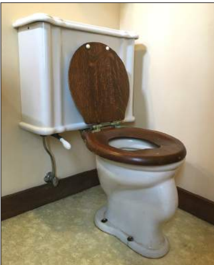
After many years and many repairs, hairline cracks in the ceramic signaled the retirement of what was purportedly the "oldest toilet in Oberlin." On the plus side, the new fixture is far more environmentally-friendly.
