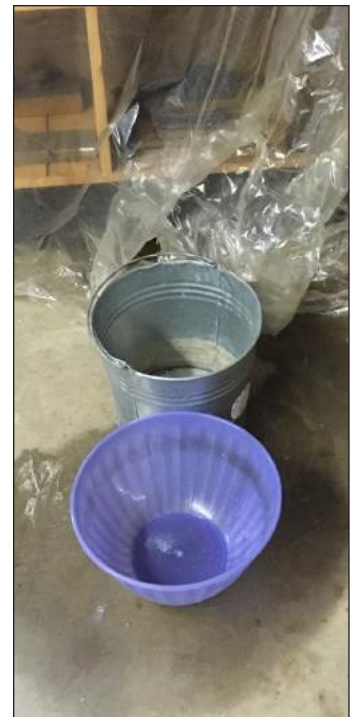
Staff were routinely checking the buildings during the shutdown, and so were able to address a pipe leak in the basement of the Jewett House before any collections items were damaged. (Thanks Turnbull Plumbing!)
